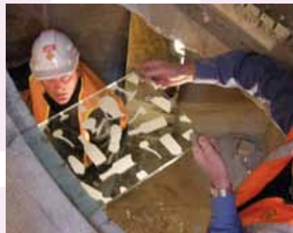
Right: Trialling the glass floor that will fit over the archaeological apertures.
